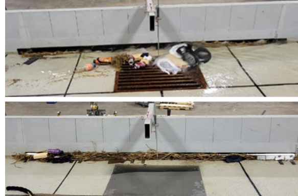
Figure 4. Debris accumulated on barrier screens following simulated debris testing.
